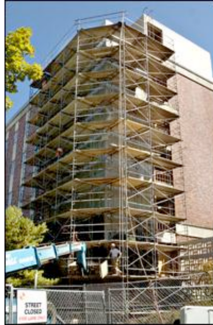
Casey Campbell | Gazette-Times Three corners of Nash Hall at Oregon State University will be stabilized as part of a $1.6 million seismic upgrade of the building. The project should be completed by fall term.
